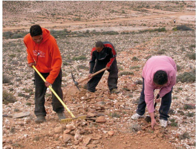
Photo 4: Members of the Griqua Community install the developed restoration treatments on the farm Ratelgat in the Succulent Karoo in September 2004. Photo: Ute Schmiedel.
